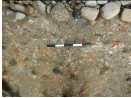
Image 4. Close view of the building's floor that has been embedded in a beachrock formation.
